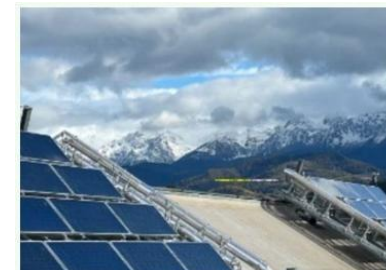
For CCIAG in Grenoble (FR) a booster station on a client rooftop
