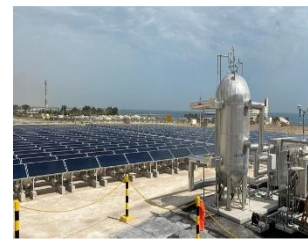
For Aramco (KSA) boiler fw preheating for an oil facility
