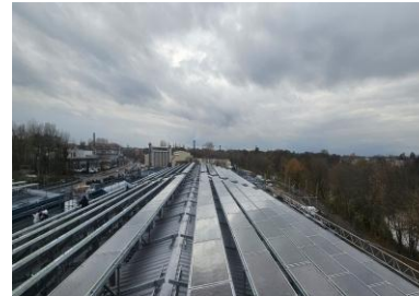
For Fernwärme Teltow (DE) a multi-rooftop distributed solar plant
