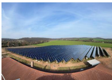
For Stadtwerke Sonderhausen (DE) a utility scale solar plant
